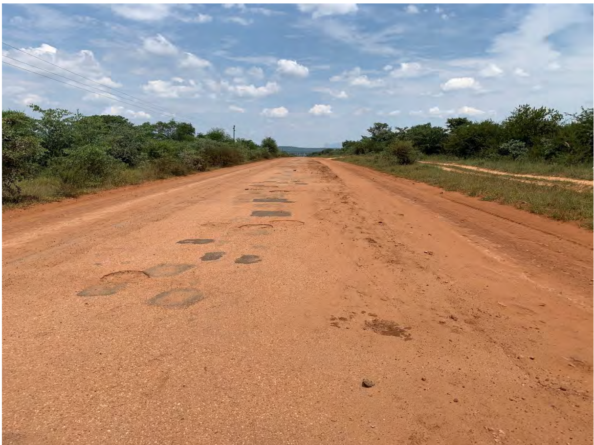
Plates 2-1: The current conditions of the road proposed for rehabilitation.
