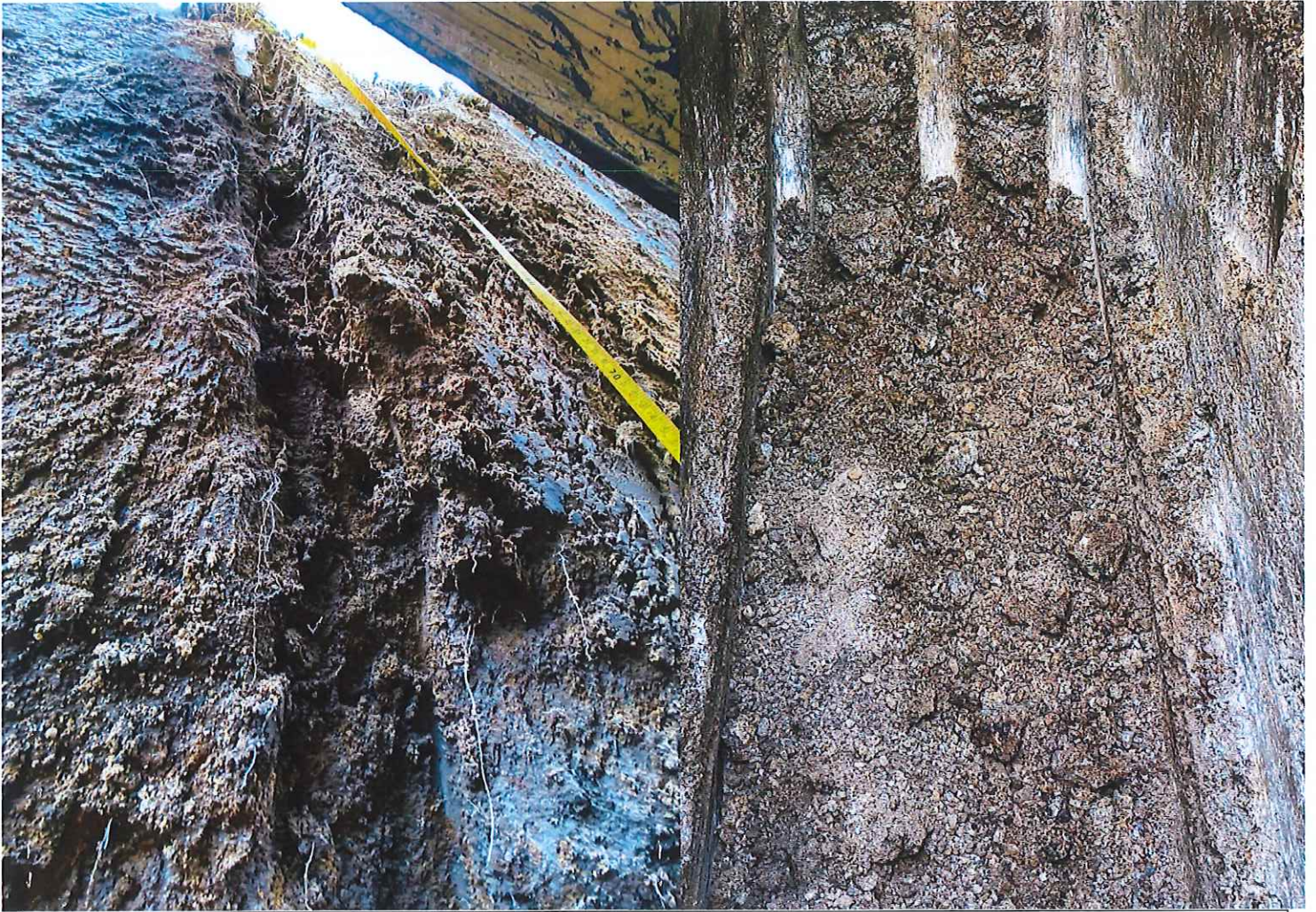
Typical alluvium transported and pedogenic soils shown from the bottom of a test holes (top left) and residual quartz porphyry horizon (right) encountered
