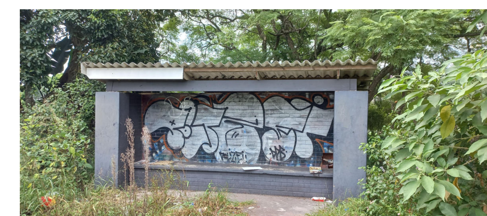
3. EXISTING COVERED SEATING STRUCTURE 2 (UNLAWFUL WORK)
