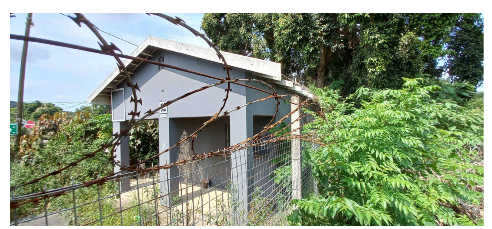
1. EXISTING TICKET OFFICE (UNLAWFUL WORK)
