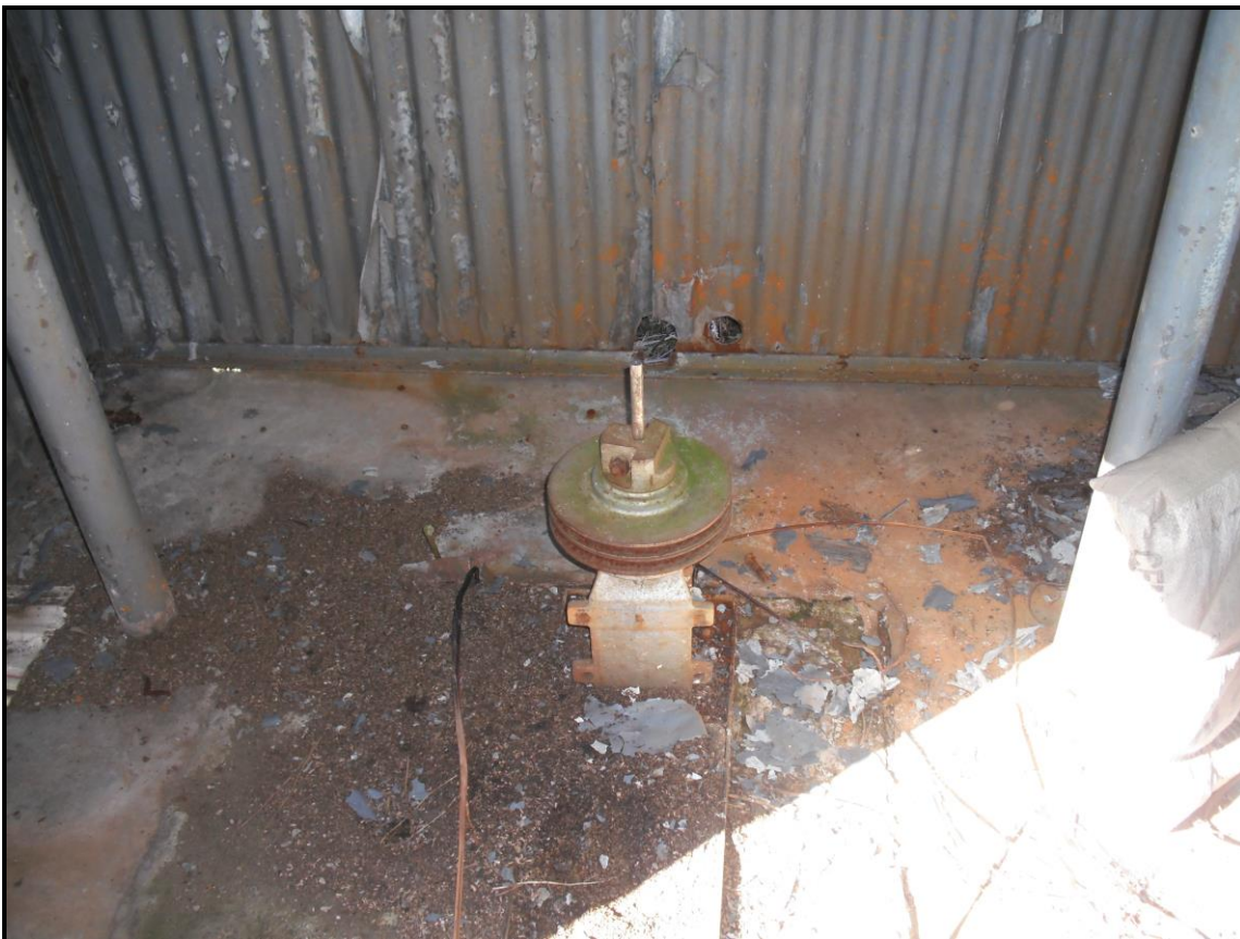
Figure 3: Borehole GBH1 previously used for water supply to Gods Window.
