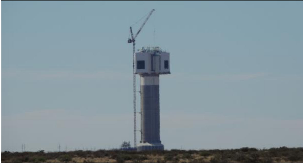
Figure 6-23: View of Khi Solar One under construction as seen from the N14
