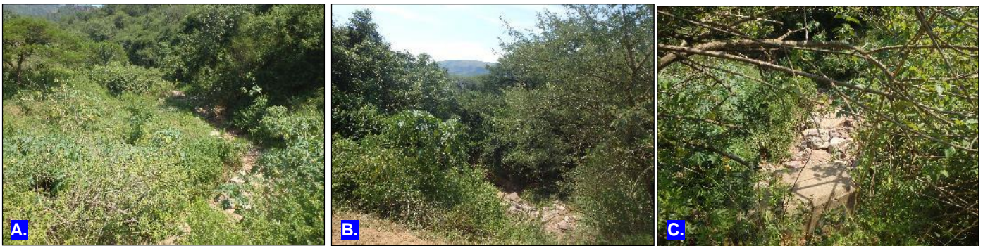
(a): Upstream of RC1. (b): Downstream of RC1. (c): A culvert upstream of RC1.
