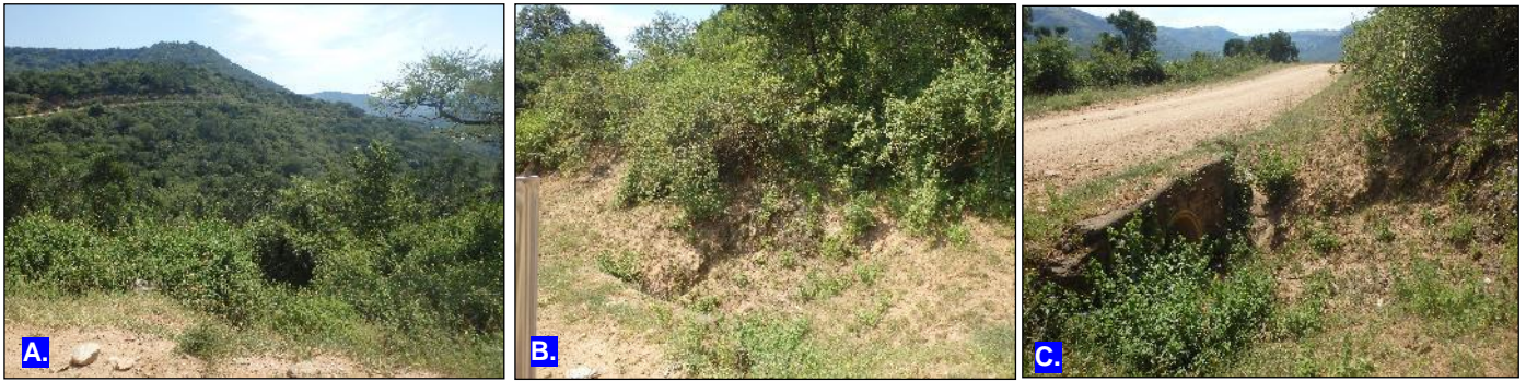
(a): Downstream of RC3. (b): Upstream of RC3. (c): A culvert situated upstream of RC3.
