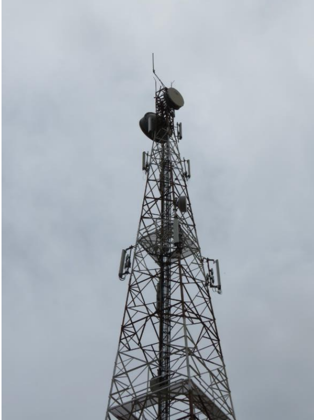
Figure 6: Typical telecom tower
