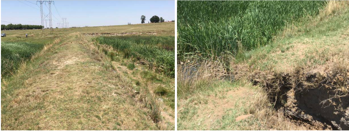
Figure 3.5: The dam wall and broken area.
