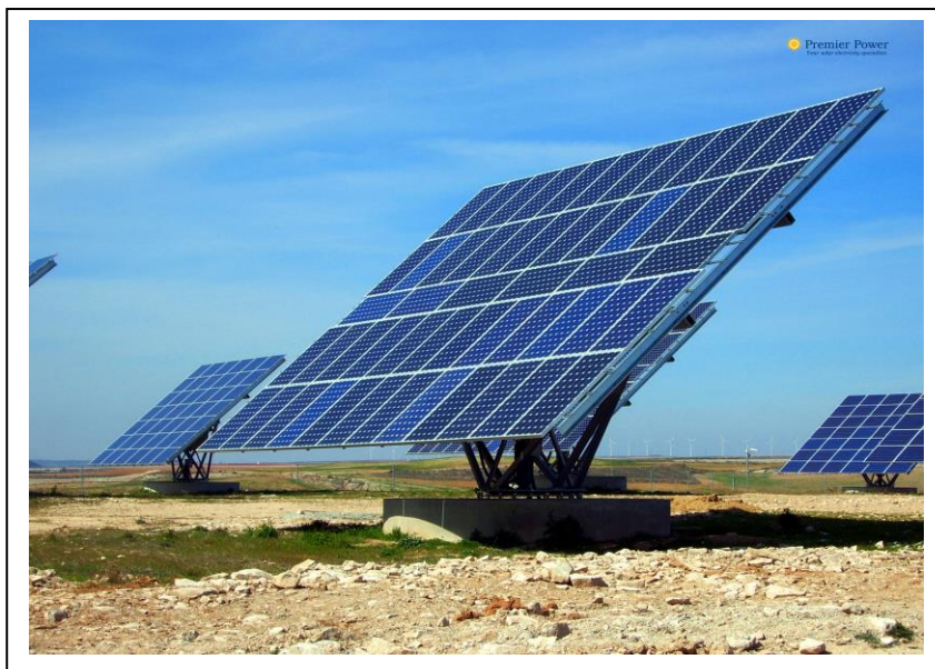
Figure 2.3: The support structures elevate the panels and allow for single axis tracking of the sun for increased efficiency (Source: Gigaom)
