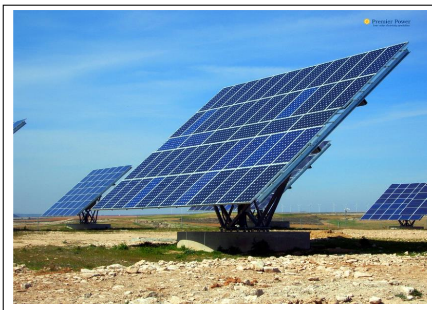
Figure 2.3: The support structures elevate the panels and allow for single axis tracking of the sun for increased efficiency (Source: Gigaom)
