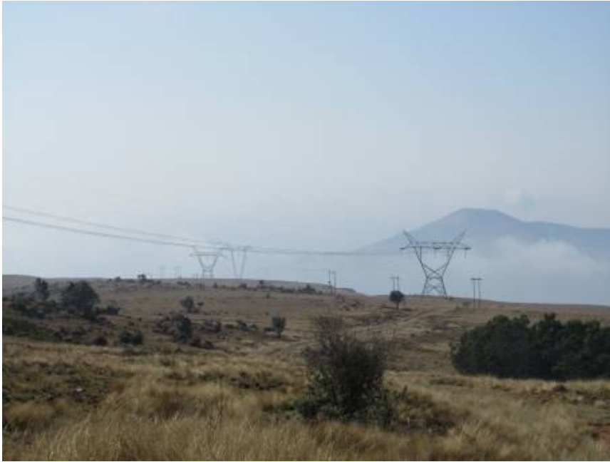
An existing HV line running along a ridge above Bosloop SS. All options are proposed to follow this line up the mountain from Bosloop SS, heading north.
