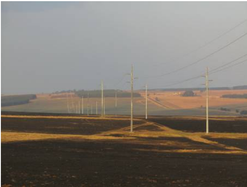
New lines being constructed with monopoles in the north of the study area. Much of the grasslands were burnt.
