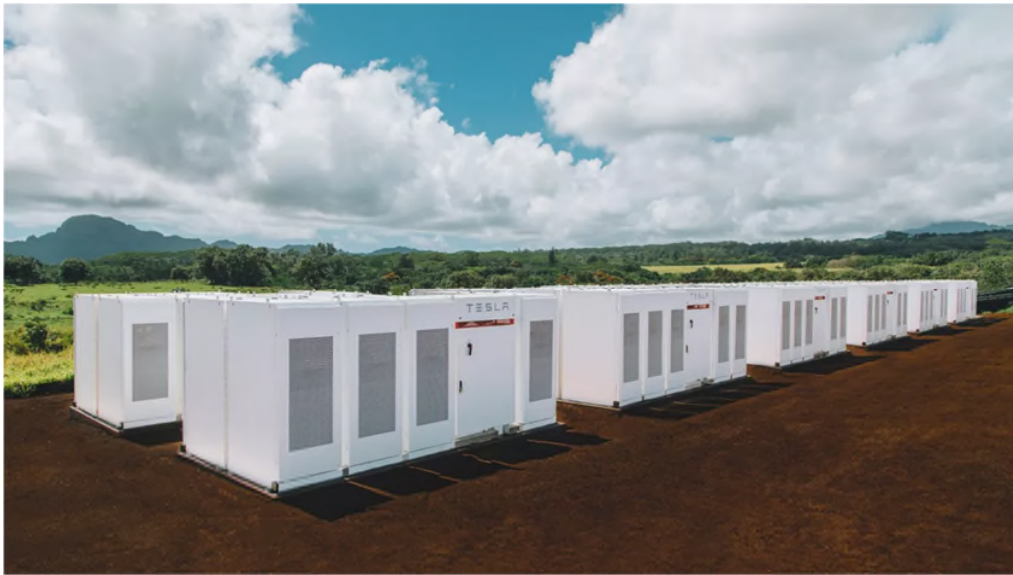
Figure 2.6: Illustration of battery storage units installed by Tesla (Source: fastcompany.com).
