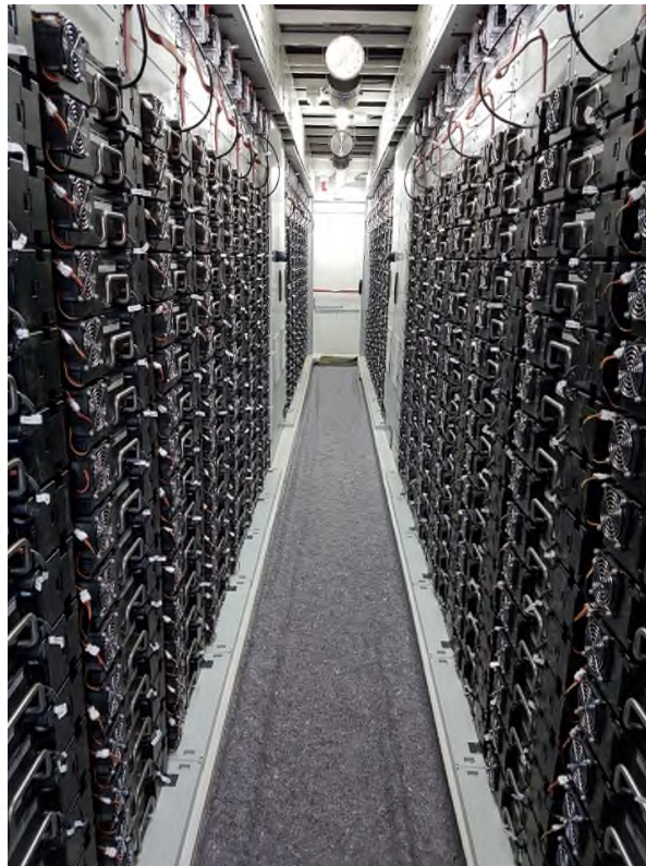
Figure 2.5: Li-Ion BESS internal design and implementation of a container used within a BESS (Source: Enel Green Power).
