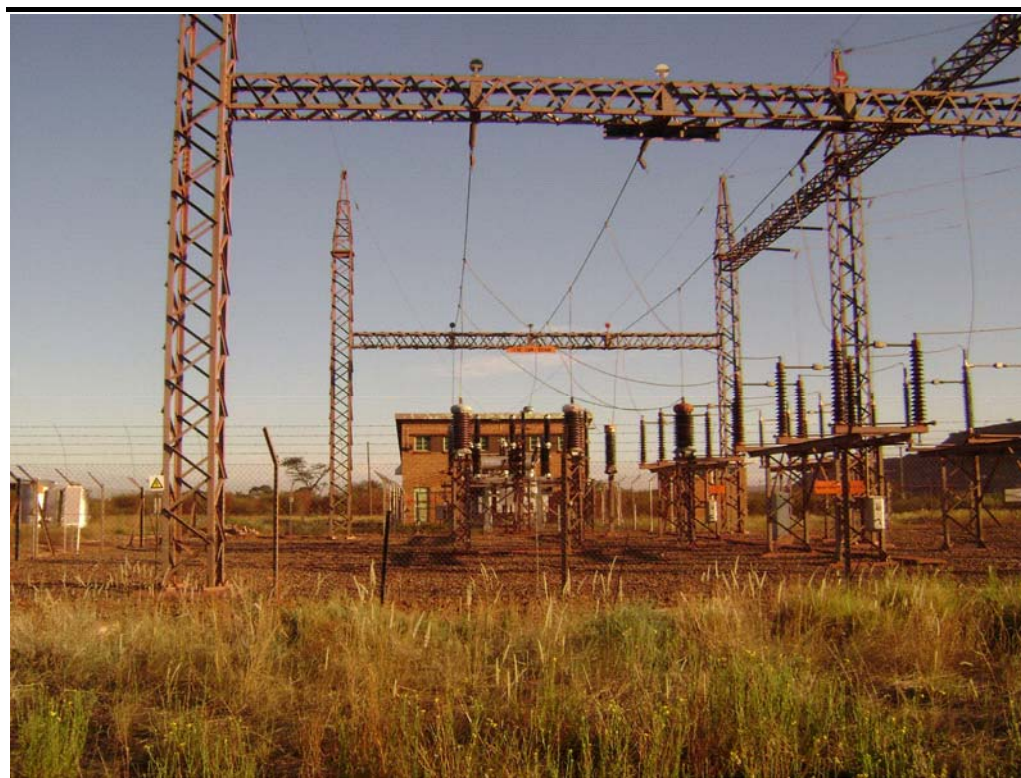
Figure 4.5 Eskom outdoor equipment (Sishen Substation)
