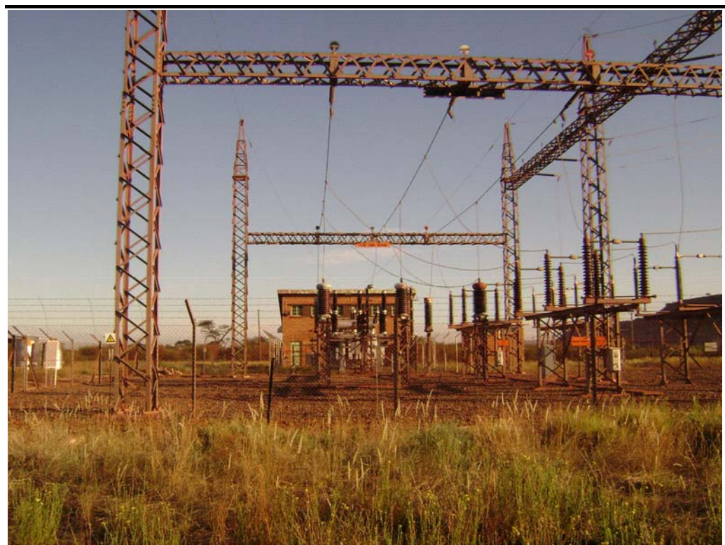
Figure 4.5 Eskom outdoor equipment (Sishen Substation)
