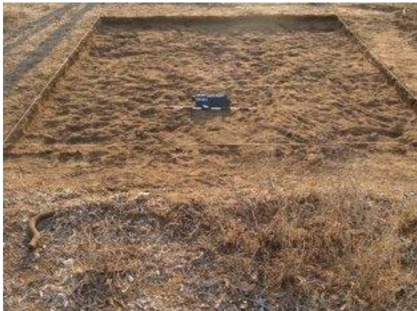
Figure 3: Excavation 1 complete. The soil was very hard, making the leveling of the excavation difficult
