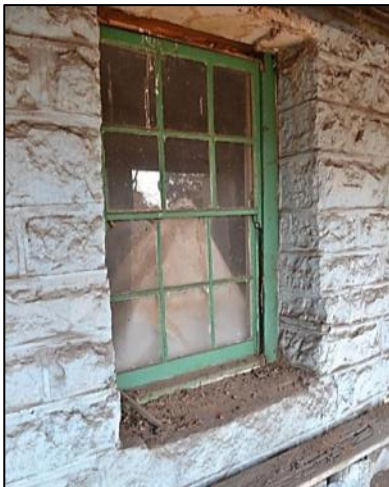
Figure 17. One of the few sash windows that have remained intact on the front verandah.
