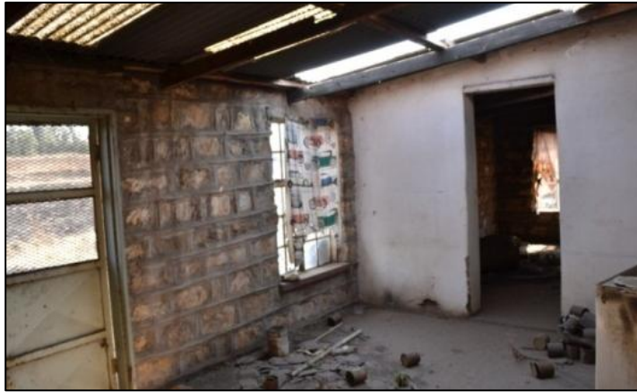
Figure 22. Closing of the open stoep at the back of the dwelling. The stoepkamer was closed with plastered brick walling.
