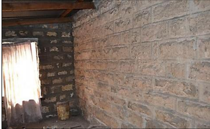
Figure 21. Original back wall of the dwelling with later additions closing the back stoep that used to be an open space.
