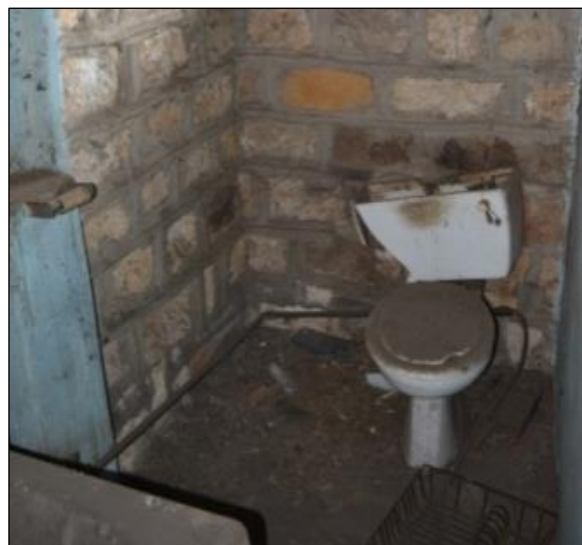
Figure 23. Crude addition and closing of the privy that was added on the back stoep of the original dwelling.
