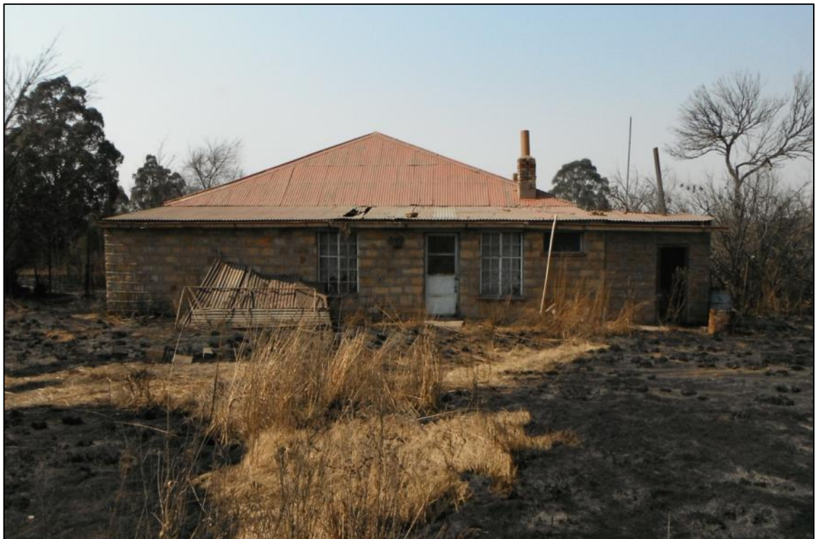
Figure 6 – Western facade of Building A. The annex in the front includes a bathroom.
