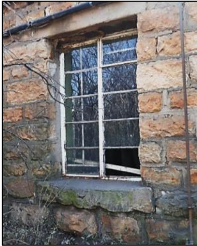
Figure 16. No exceptional stone work appears around the windows whereas the sills were dealt with in a direct and unrefined way.
