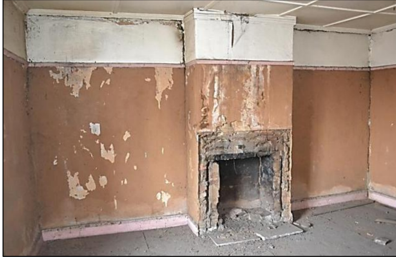
Figure 18. Remains of clay plastering in the principal lounge. The mantelpiece has been removed.
