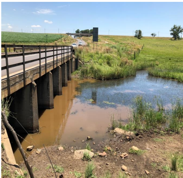
Crossing of the pipeline over the Klippoortjiespruit along the bridge
