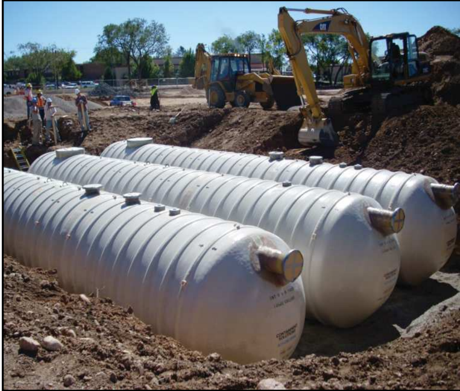
Figure 6: Sewerage Conservancy Tanks
