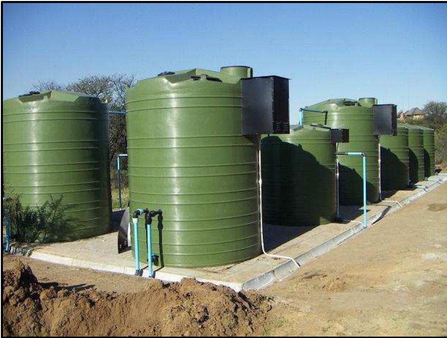
Figure 2: Non-Mobile Sewerage Treatment Package Plant
