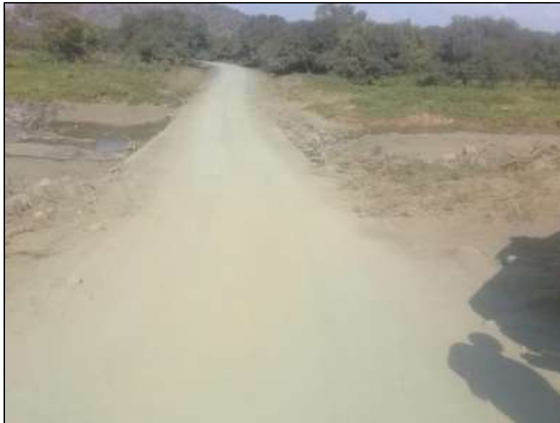
Photograph 6: Showing the existing road conditions associated with the Kwabovu structure located along P176.
