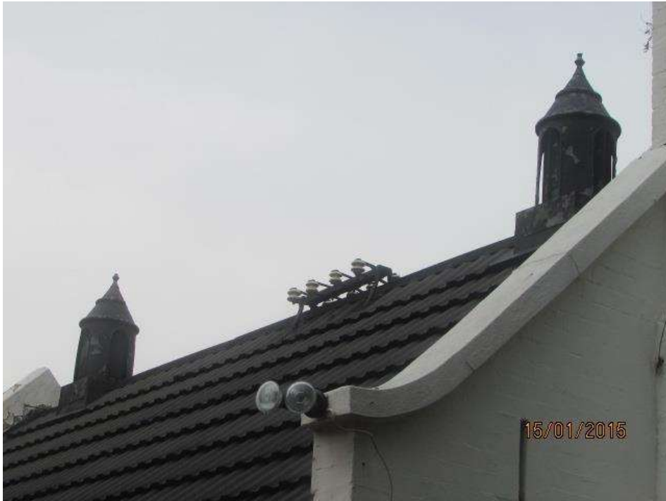
Figure 27: A closer view of Victorian-style features on the roof of the house.
