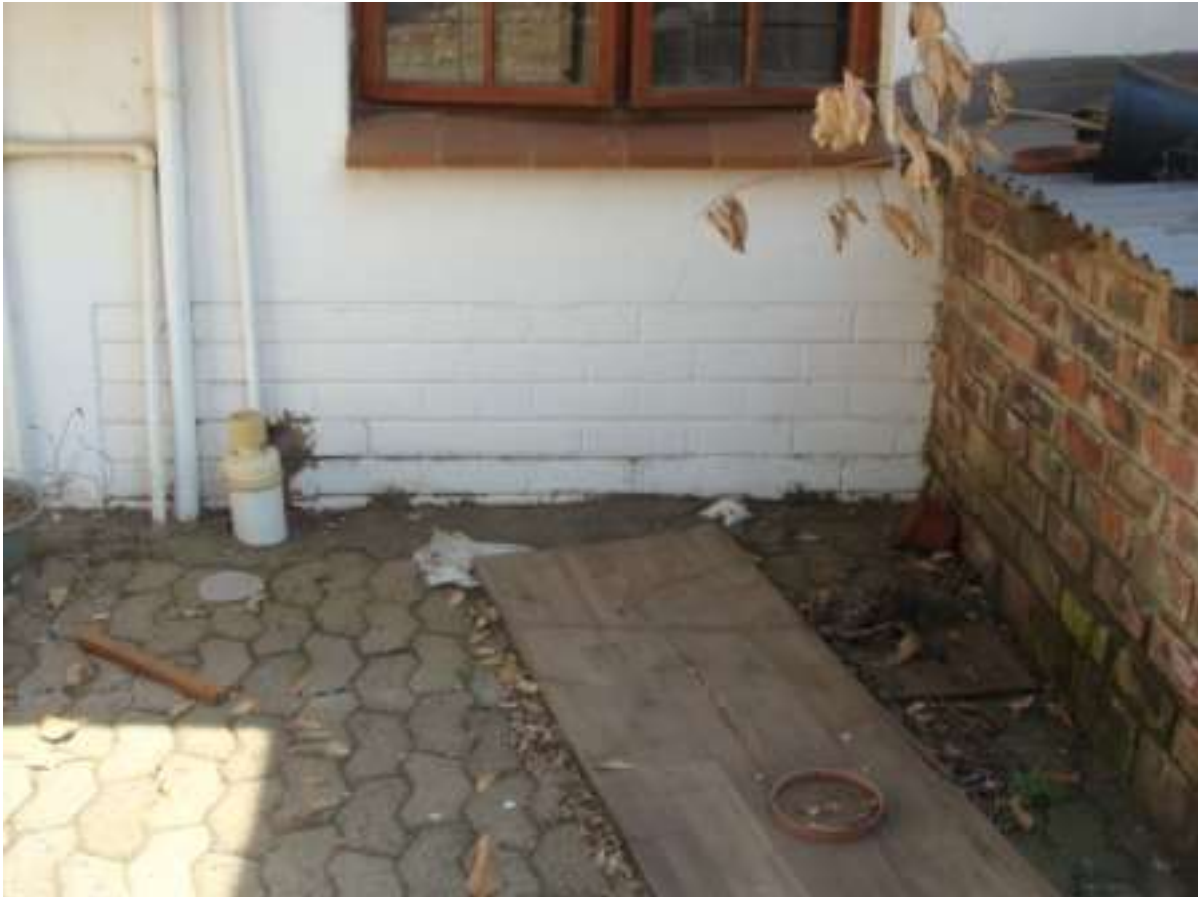
Figure 12: A section of plastered over bricks that could be the remnants of the original 1949 structure.
