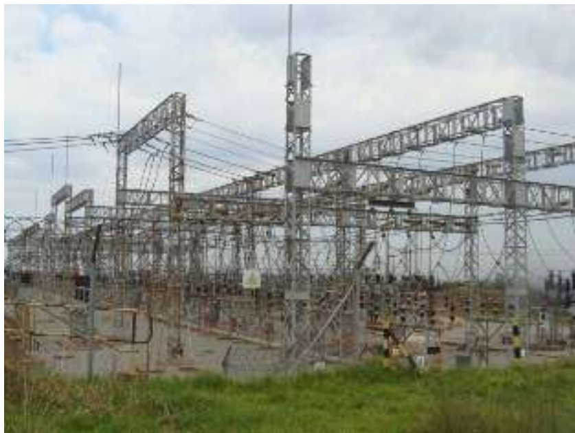
Figure 5: Another view of substation infrastructure.
