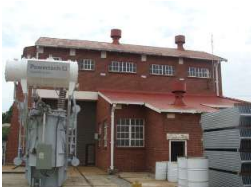
Figure 7: The main Control Room/Rotary Room/Distribution station.
