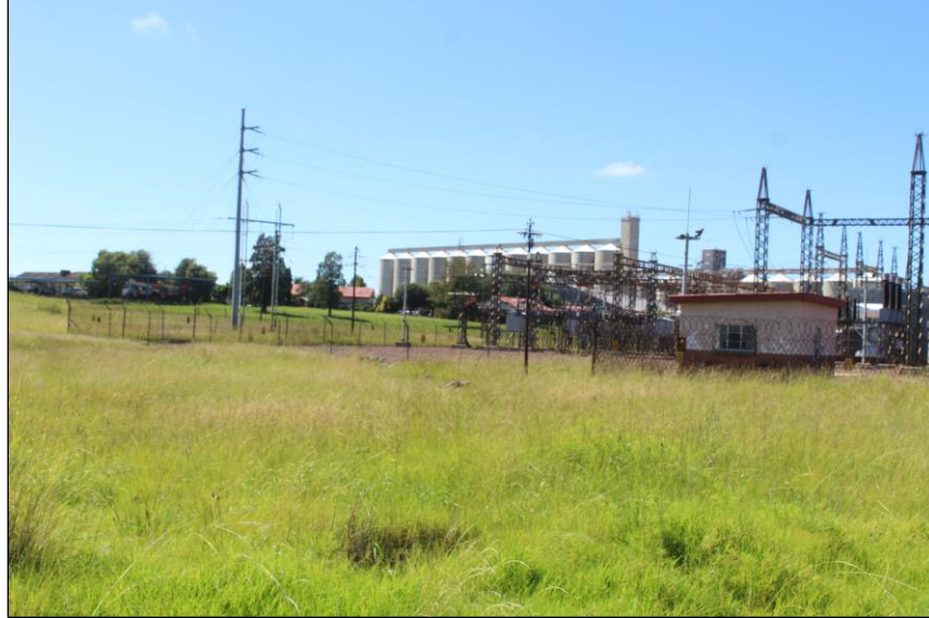
Figure 2: Power will be drawn from an existing substation on the northern outskirts of Bethal
