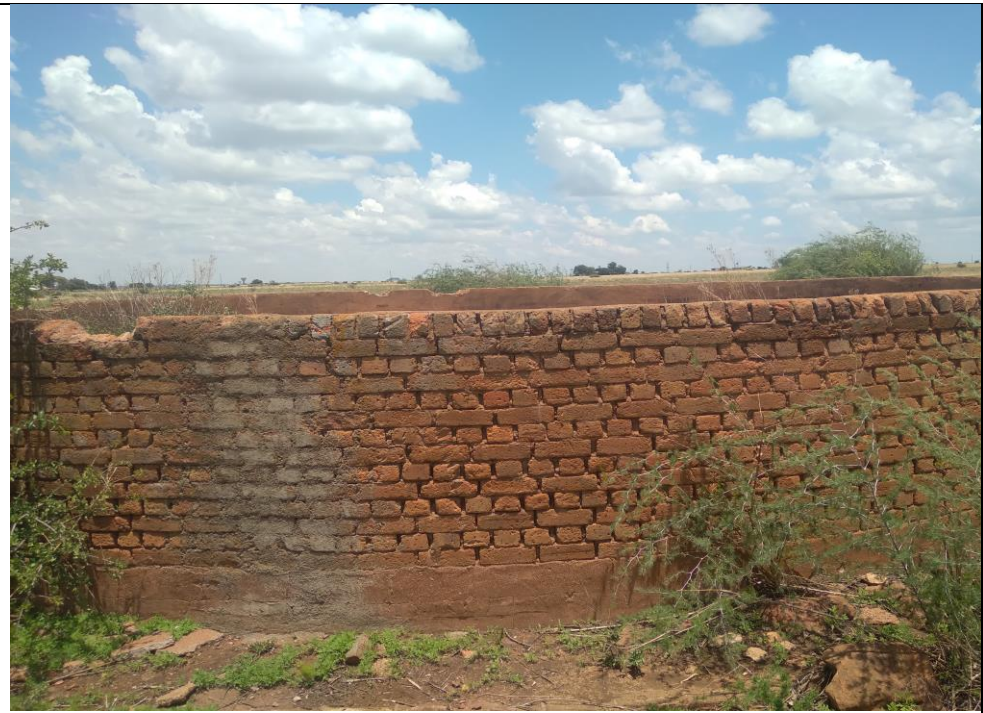
Figure 12: Outside view of the tank. Note that the tank might be over 60 years old but still does not have any heritage or architectural significance and may be demolished as it has been recorded through this report.
