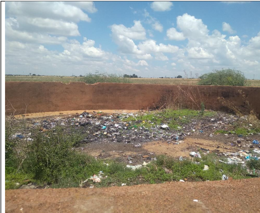
Figure 11: View of an old disused water tank now being used as a rubbish dumping site within the proposed development site
