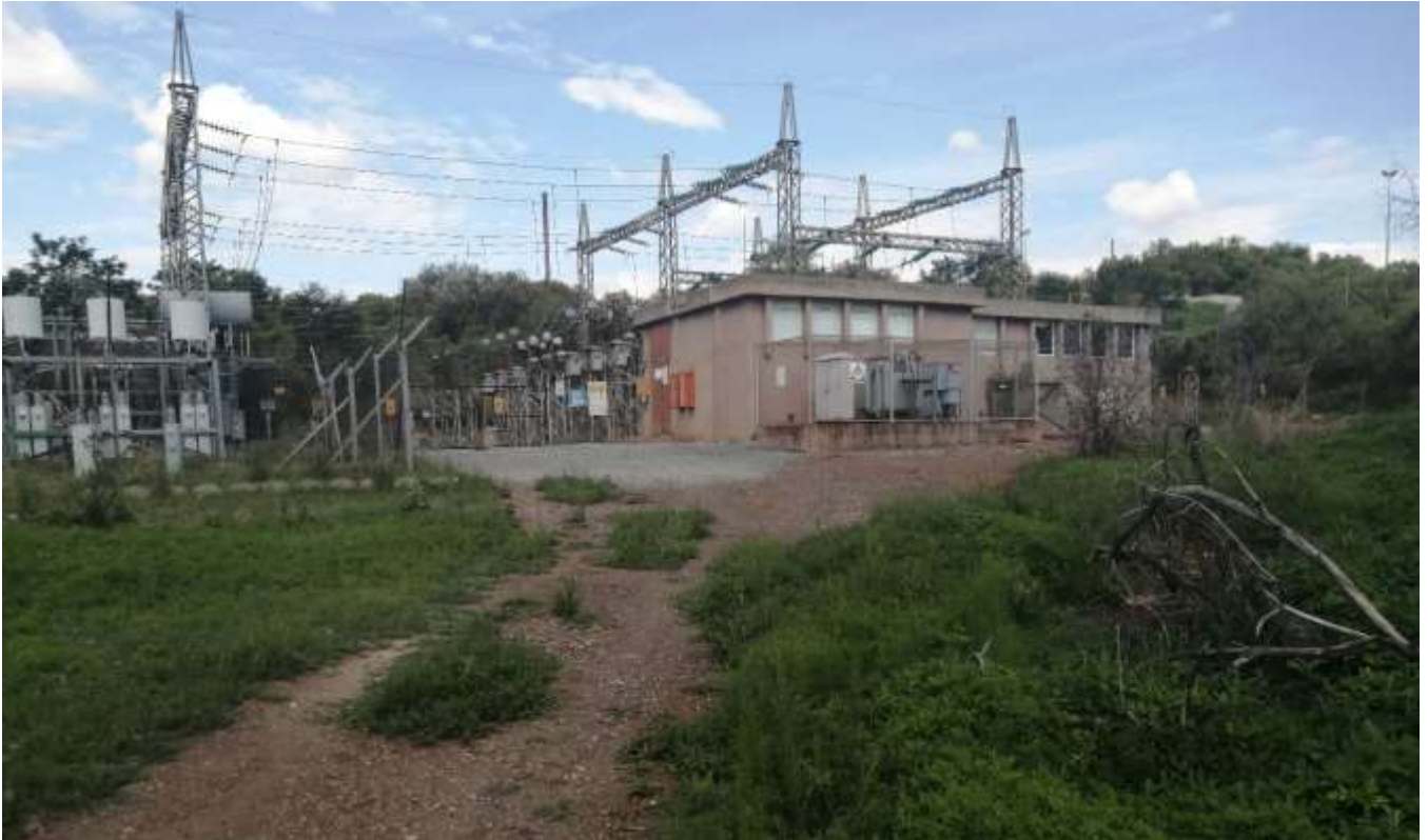
Plate 16: Showing existing Safari substation
