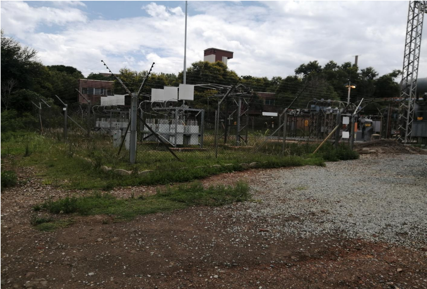
Plate 1: Showing the substation associated with the proposed development.
