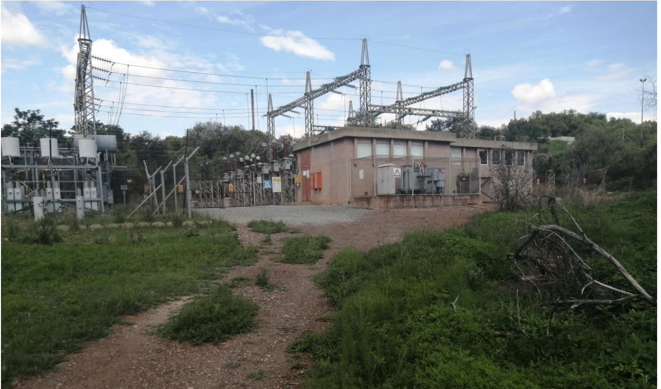
Plate 16: Showing existing Safari substation
