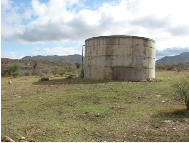
Figure 9 – View of the existing reservoir where the proposed 355mm pipeline will start.
