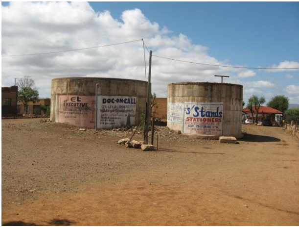
Figure 5 - View of the existing reservoir where the proposed 140mm pipeline will start.
