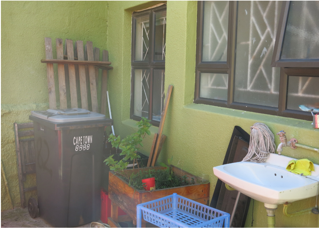
Existing storeroom and bathroom at the back of the site demolished. These structures were added in 1980.
