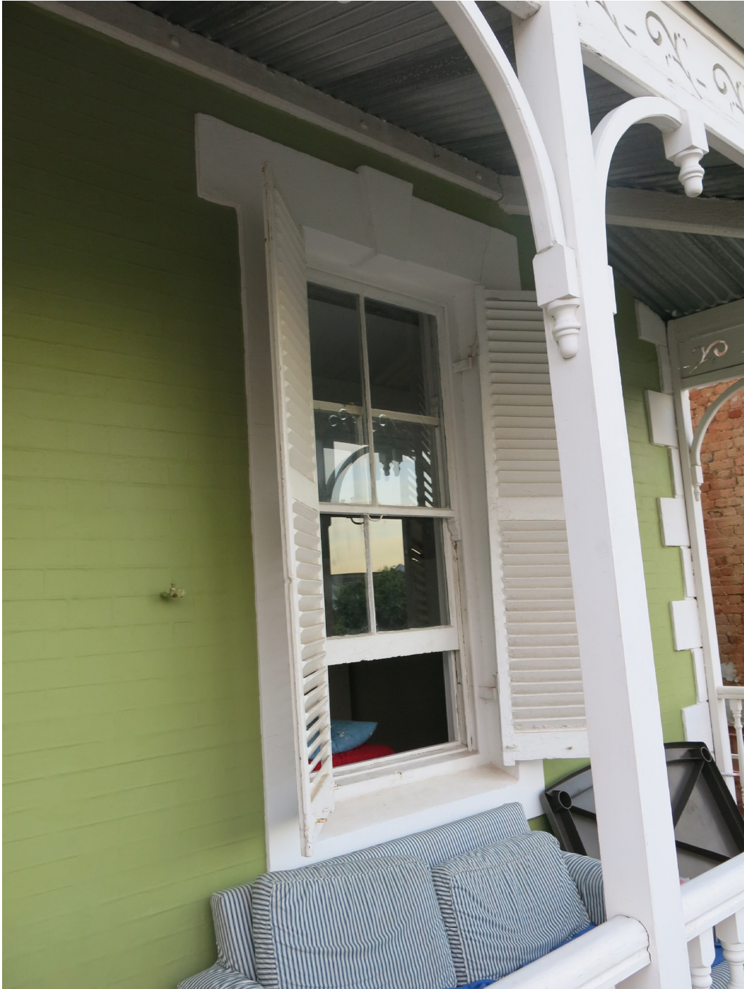
Sash windows, timber shutters and original timber balustrading to be repaired and retained.
