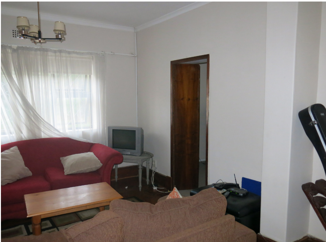
Existing lounge. New bathrooms built in this zone, with a new wall on the line of a previous wall. (nibs, beam and foundations visible)
