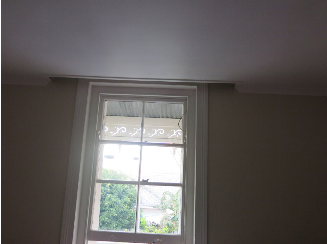
Existing ceiling removed to reveal higher original timber ceiling. Timber ceiling to be repaired where possible.
