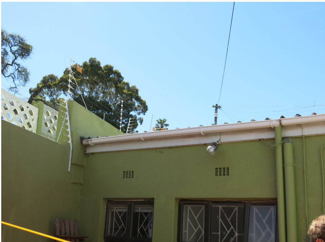
Existing storeroom and bathroom at the back of the site demolished. These structures were added in 1980 and has no historical, or other value. Once removed, North Eastern sunlight can penetrate the new outside area /courtyard outside the new sliding door.
