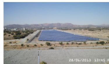
7MW RustMo1 Solar Farm near Rustenburg - Operational
