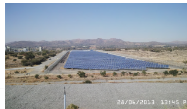
7MW RustMo1 Solar Farm near Rustenburg - Operational
