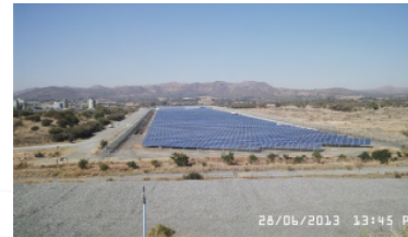
7MW RustMo1 Solar Farm near Rustenburg - Operational
