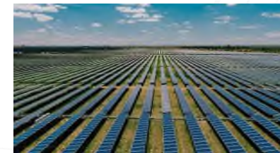
50MW De Wildt Solar Power Plant near Brits – Commenced commercial operation in January 2021
