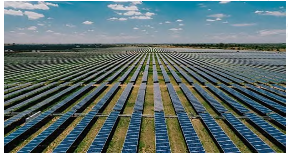
50MW De Wildt Solar Power Plant near Brits – Commenced commercial operation in January 2021
