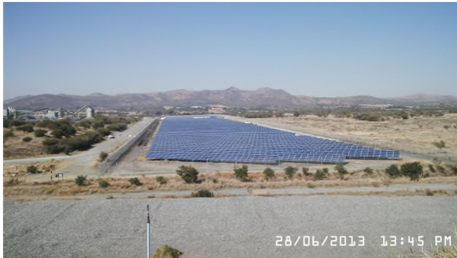
7MW RustMo1 Solar Farm near Rustenburg - Operational
