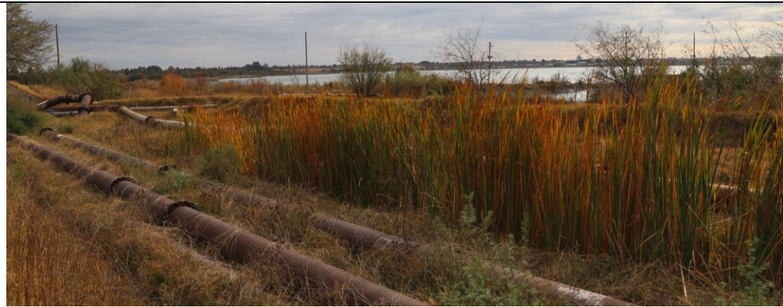
Modifications and sever degradation is evident along the shores of the Witpan.
