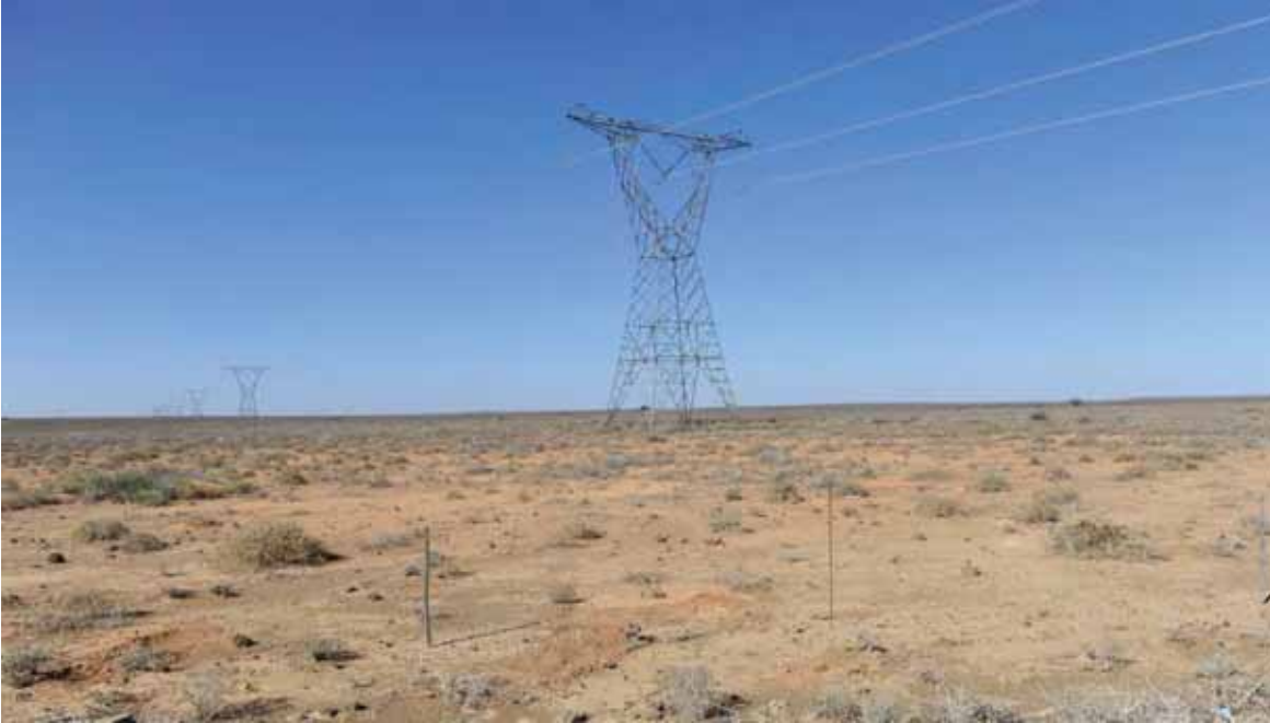
Figure 7: The existing Aries-Kronos 400kV transmission line which runs just south of the proposed development site.
