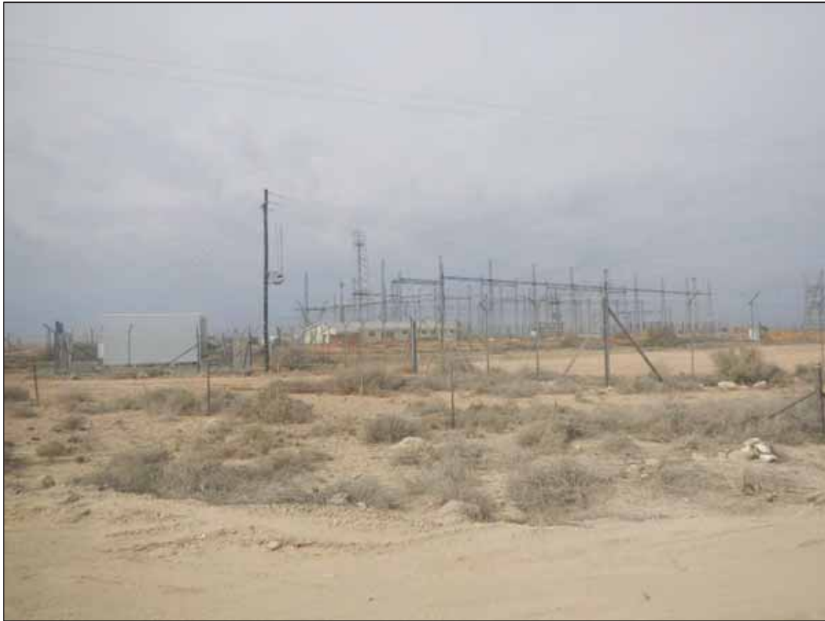
Figure 27: View of the existing Eskom Kronos Substation
