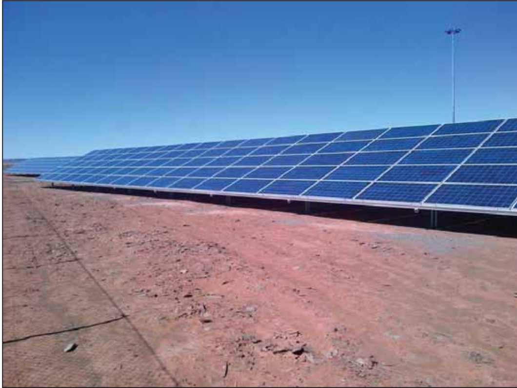
Figure 15: Photovoltaic Panels being erected near De Aar in the Northern Cape Province
