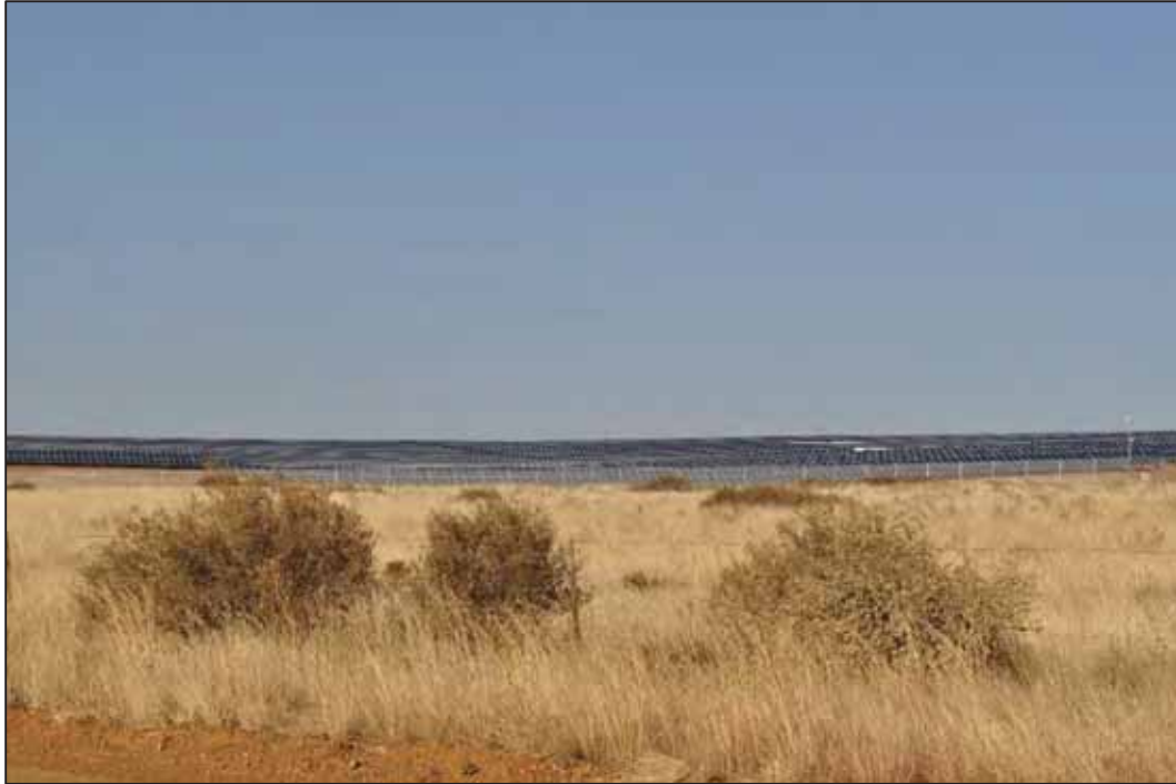
Figure 16: Photovoltaic Panels being erected near Lime Acres in the Northern Cape Province
