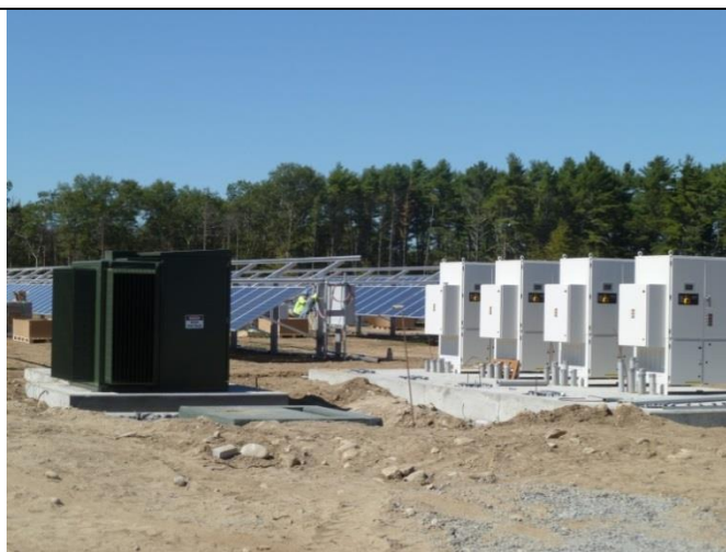
Figure 6: Inverter (Photo courtesy of BlueWave Capital SA)
