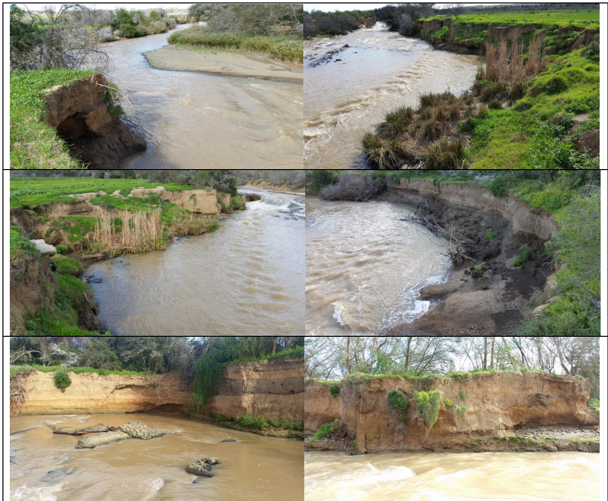
Figure 7: Erosion (rehabilitation) areas in the Skoenmakers River
