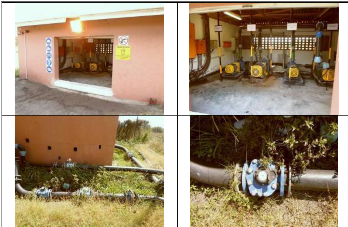
Figure 4.2.1.5(a): Photographs of the Canal Water Supply Pump Station
