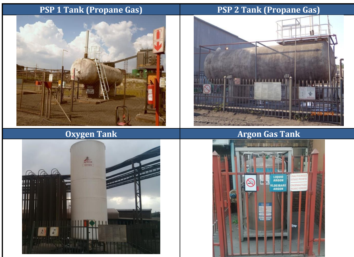
Figure 4.2.1.7(a): Photograph of the Gas Supply Tanks
