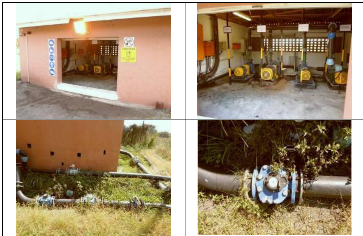
Figure 4.2.8.1(a): Pump Station Infrastructure
