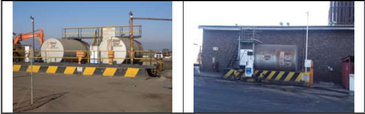
Figure 4.2.1.8(a): Photographs of the HERNIC Diesel Storage Areas
