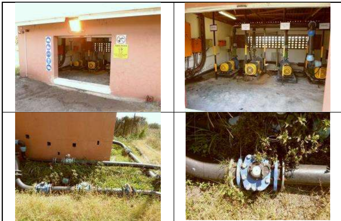
Figure 4.2.8.1(a): Pump Station Infrastructure
