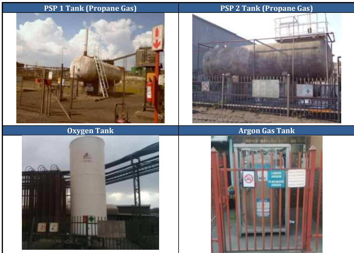
Figure 4.2.1.7(a): Photograph of the Gas Supply Tanks
