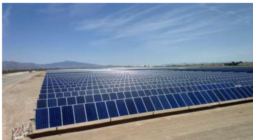
Figure 5: Illustration of tracking PV technology panels
