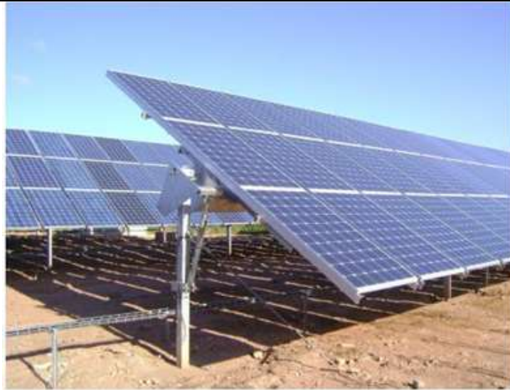
Figure 3: PV panels installed
