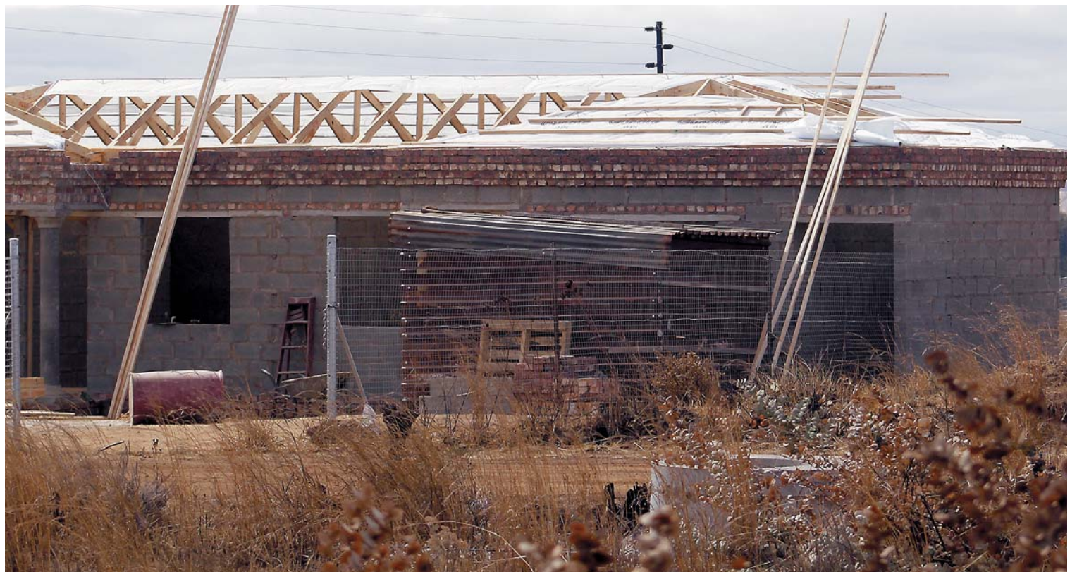
Some Middle Class Earners committee members have begun building on the allocated land near the N11 Hendrina road.
