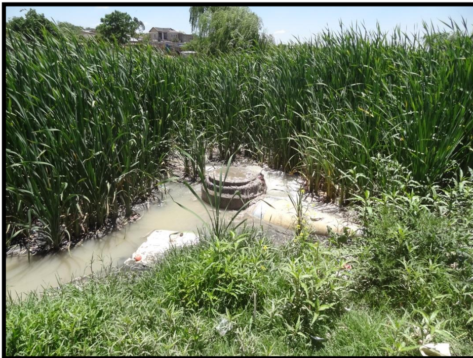
Photo 10: Sewer leaking into the stream
