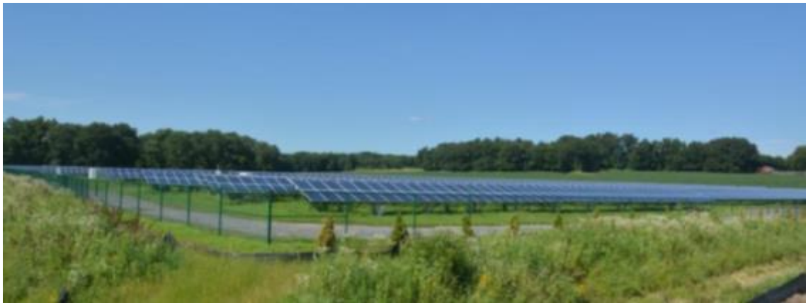
Plate 1, PV array viewed from approximately the same ground level as the array. Note the array appears as a linear dark element in the landscape
