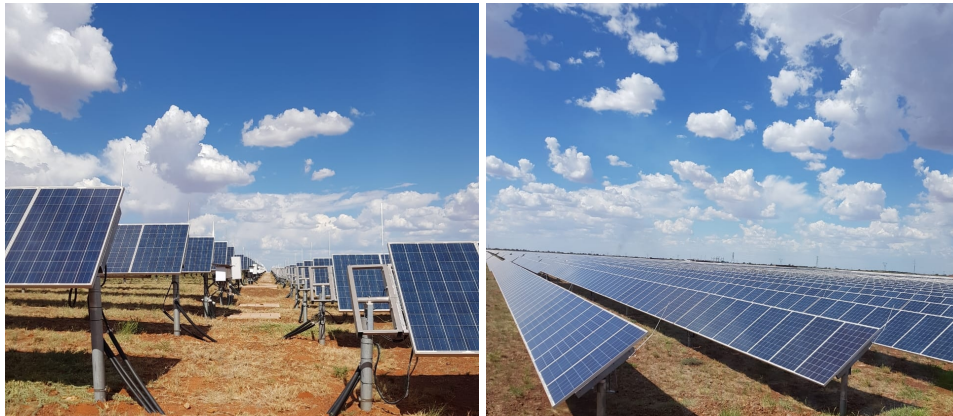
Figure 1: Solar PV facility (Courtesy of Building Energy South Africa (Pty) Ltd)
