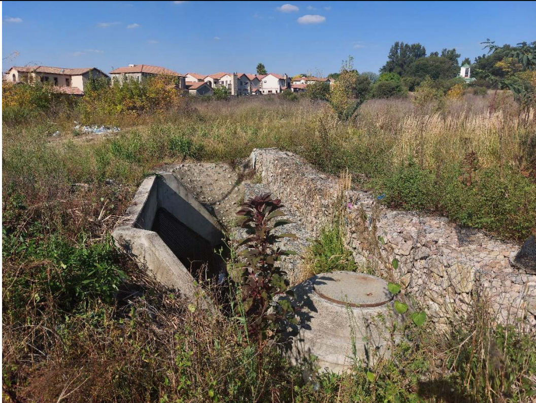
Culvert to manage stormwater across Frederik Road
