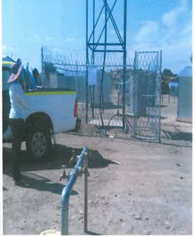
Silver City Water Collection Point (West of Sterkstroom River)
