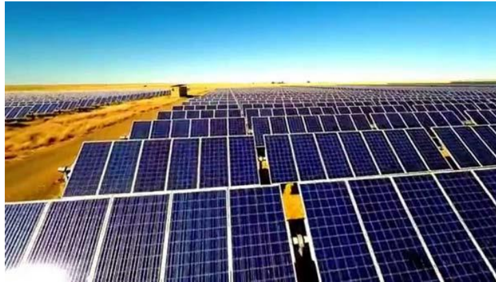
Figure 1: An example of a solar plant
