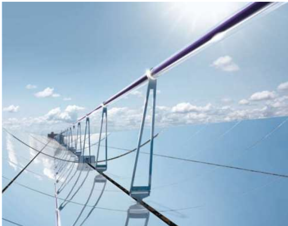
Figure 3.4: The top photograph illustrates the pipes conveying the heat transfer fluid and the bottom photograph illustrates the parabolic troughs together with the receiver tube (Source: Siemens AG)
