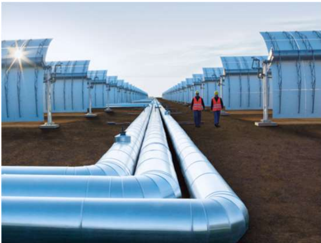
Figure 3.5: The pipes lain between the troughs convey the heat transfer fluid (Source: Siemens AG)
