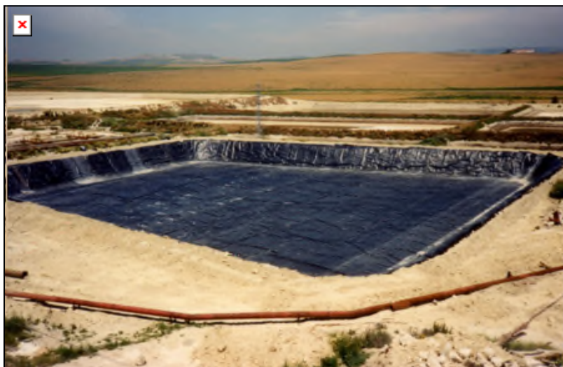
Figure 2.8 Photograph of a typical lined evaporation pond utilised for a CSP Plant
