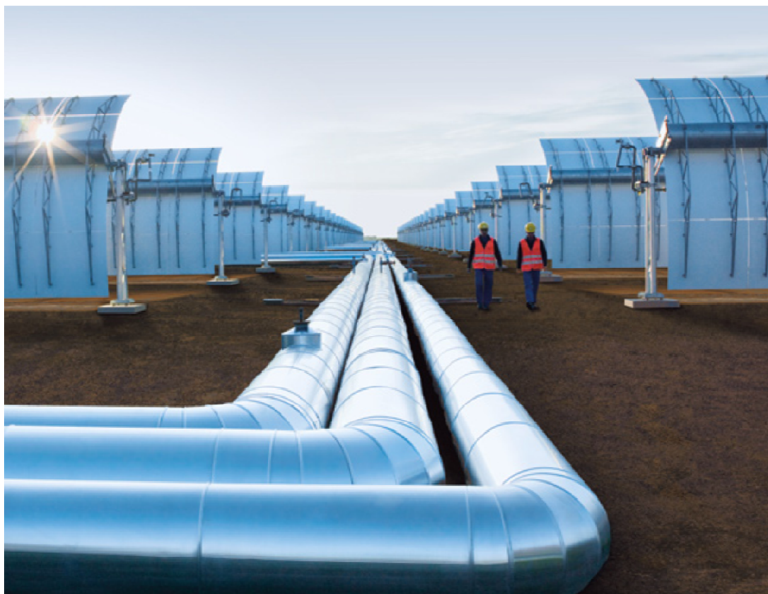
Figure 2.6: The pipes lain between the troughs convey the heat transfer fluid (Source: Siemens AG)
