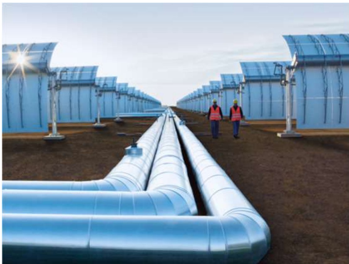
Figure 3.5: The pipes lain between the troughs convey the heat transfer fluid (Source: Siemens AG)
