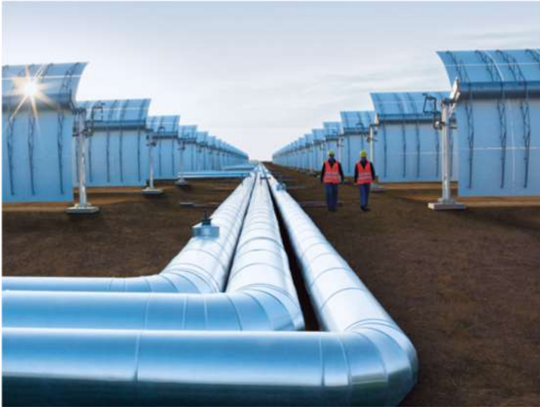
Figure 2.6: The pipes lain between the troughs convey the heat transfer fluid (Source: Siemens AG)
