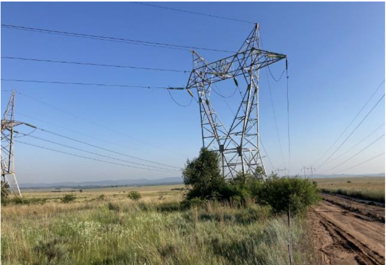
Figure 8: High voltage lines
