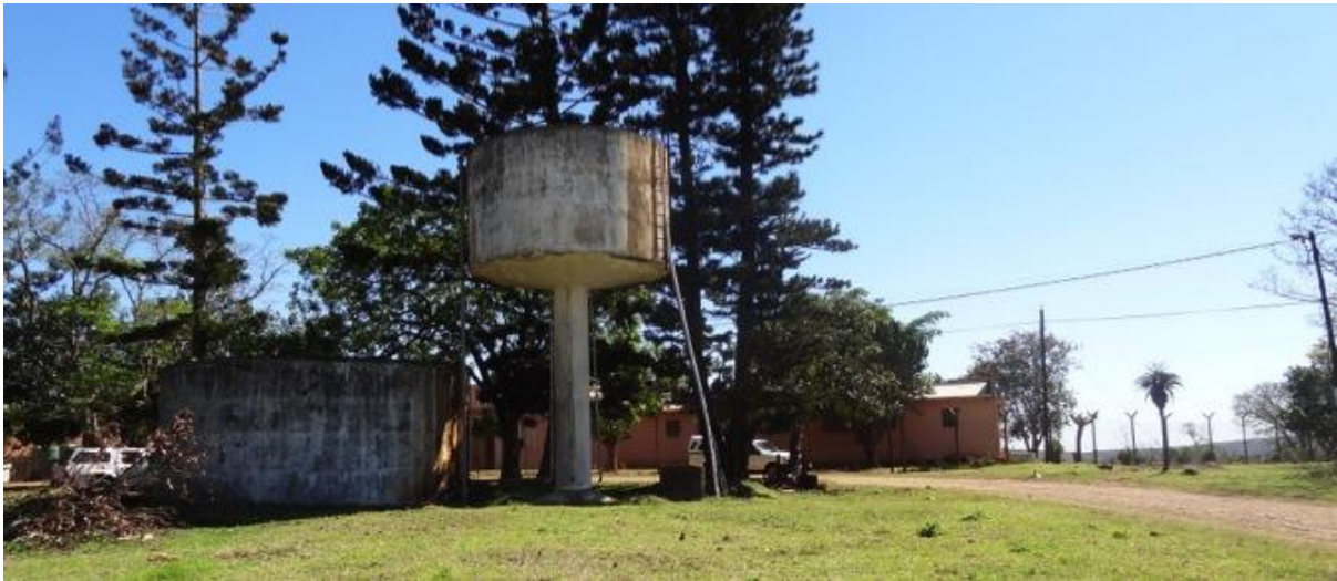
Existing water reservoir in Ingwavuma Town Centre with the Prison in the background.
