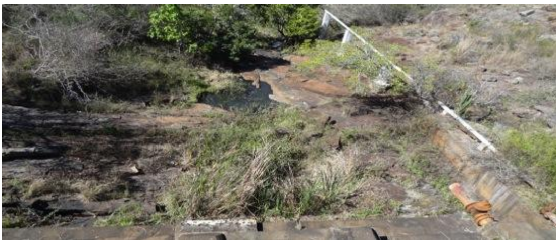
Existing water pipeline drawing water from the weir dam to feed the hospital line
